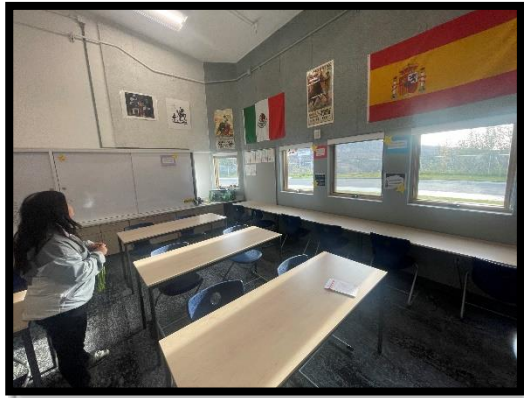
FIGURE 7. CLASSROOM 101 FIN TUBE LOCATION
