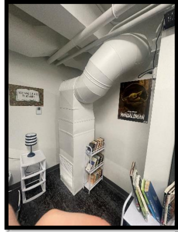
FIGURE 6. CLASSROOM 160 DUCT TO BE RECONFIGURED
