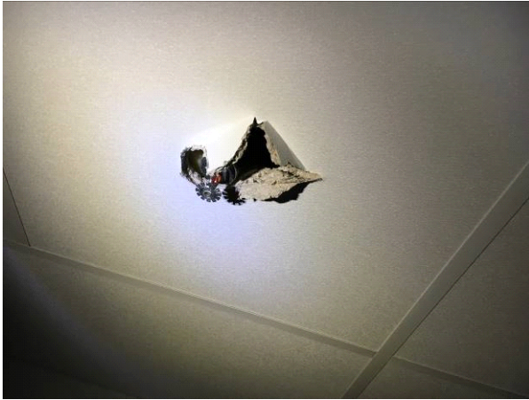
Figure B9. Sprinkler Head without Adequate Ceiling Clearance, in Room 302A
