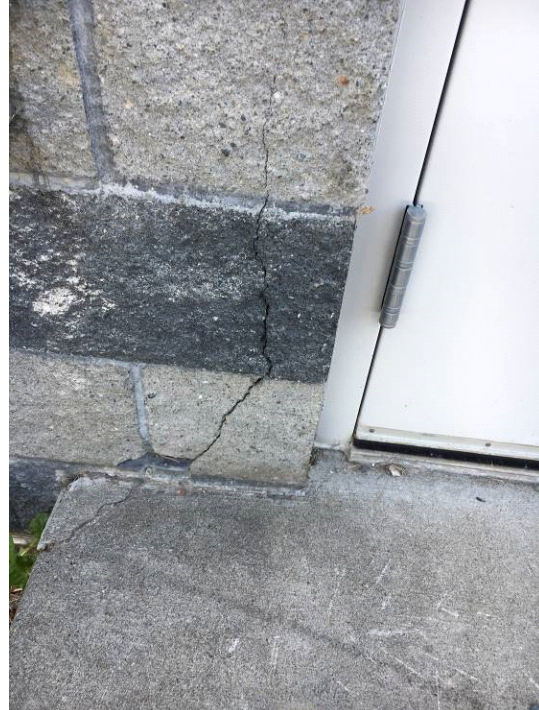
Figure B8. Damaged Façade CMU, Adjacent to Room 306 Exterior Door
