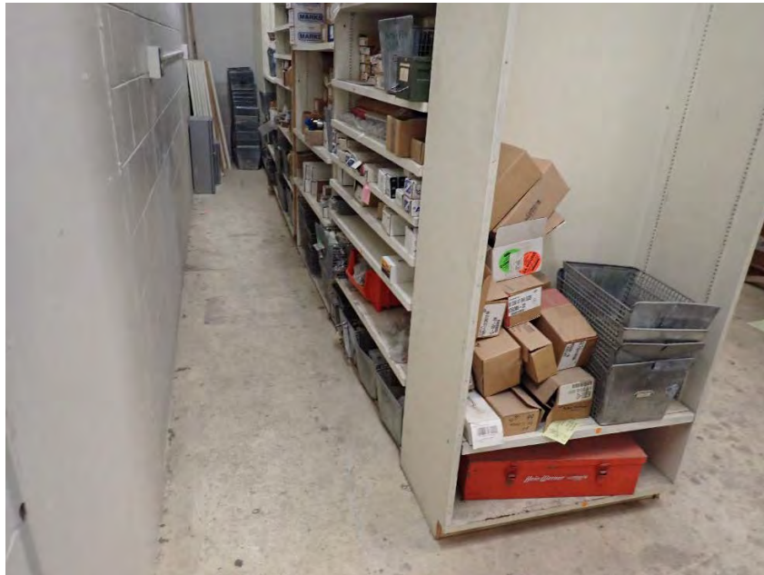
Door Shop, Unrestrained Shelves & Fall Prone Contents Figure B- 28
