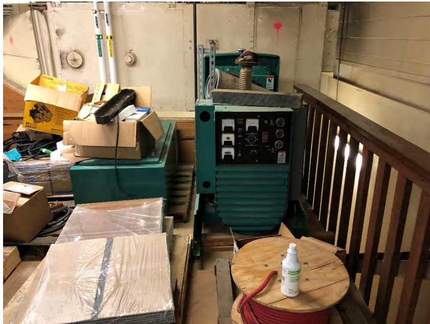
MCR Mezzanine 236, Fall Prone Contents Figure B- 58
