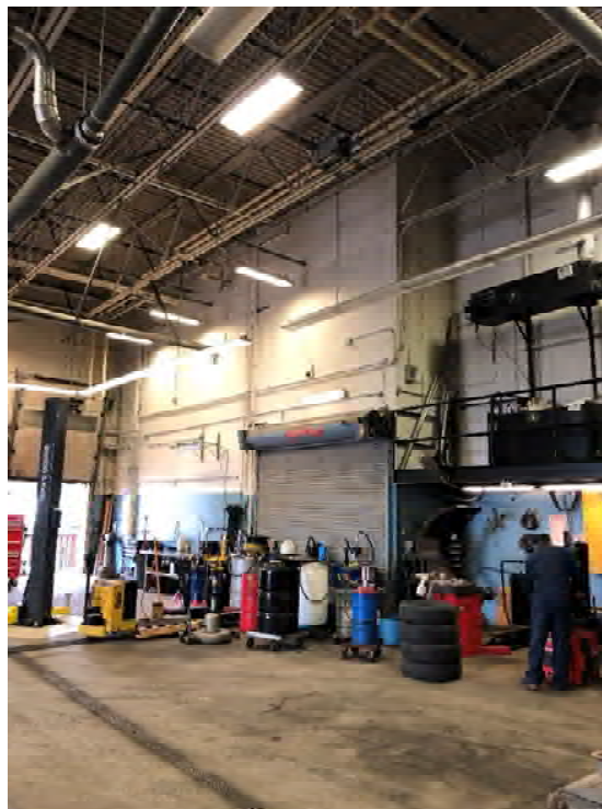
Vehicle Shop, Improperly Restrained Lighting Figure B- 48
