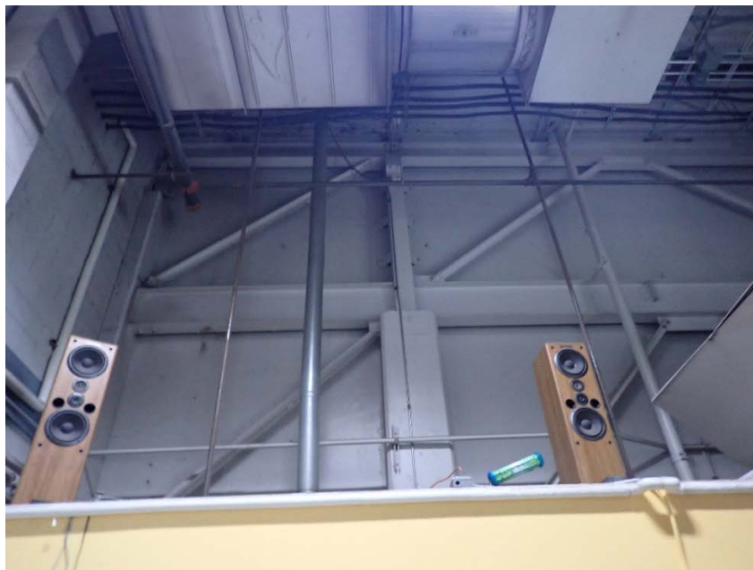
Paint Shop, Improperly Restrained Piping and Vent Figure B- 26
