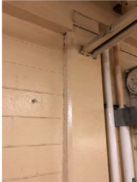
MCR Mezzanine 236, CMU Cracking Figure B- 61
