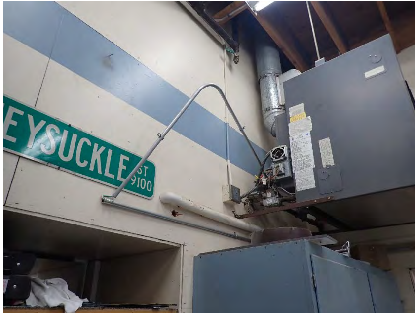
Glass Shop, Improperly Restrained Mechanical Unit
