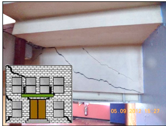
Figure 3: Life Safety (S-3) - Cracking/deflection in concrete beam, cannot be repaired.
