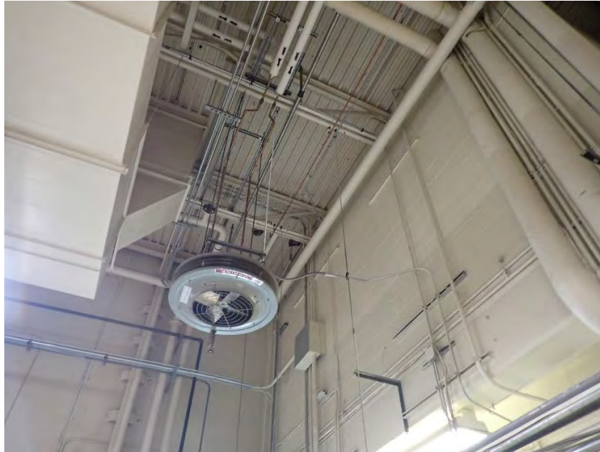
Room 105, Improperly Restrained Fan Figure B- 35
