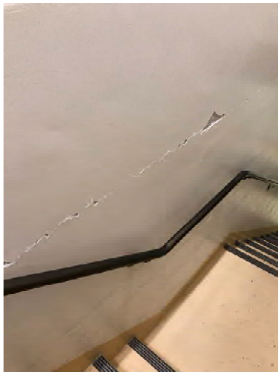
SW-3, CMU Cracking Figure B- 68
