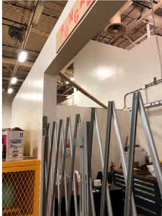
MCR Open Circulation, Partitions Improperly Restrained Figure B- 85
