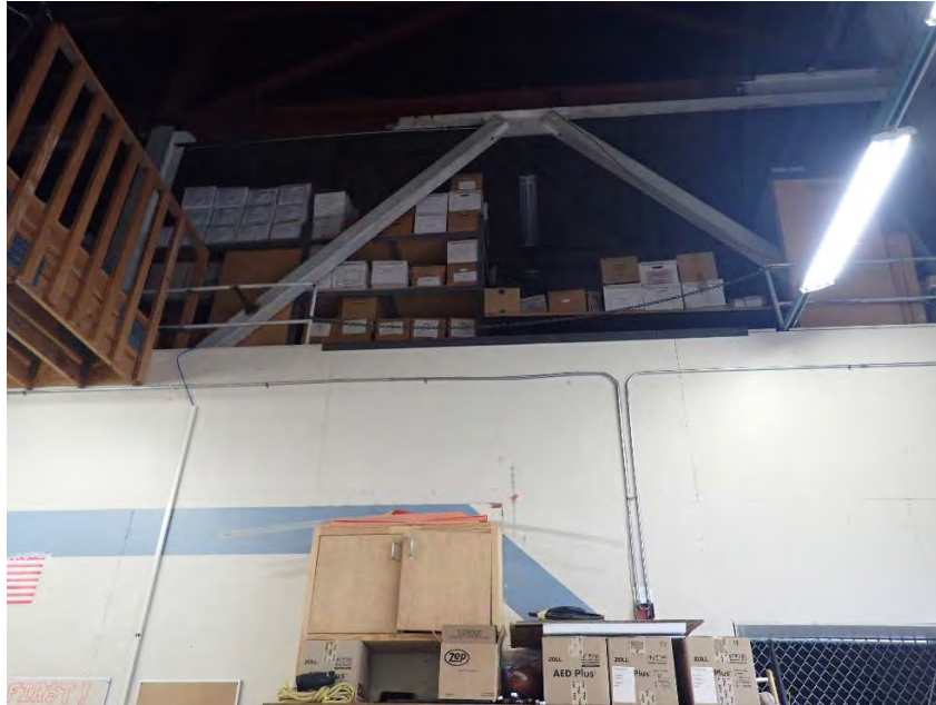
Glass Shop, Fall Prone Contents Figure B- 31
