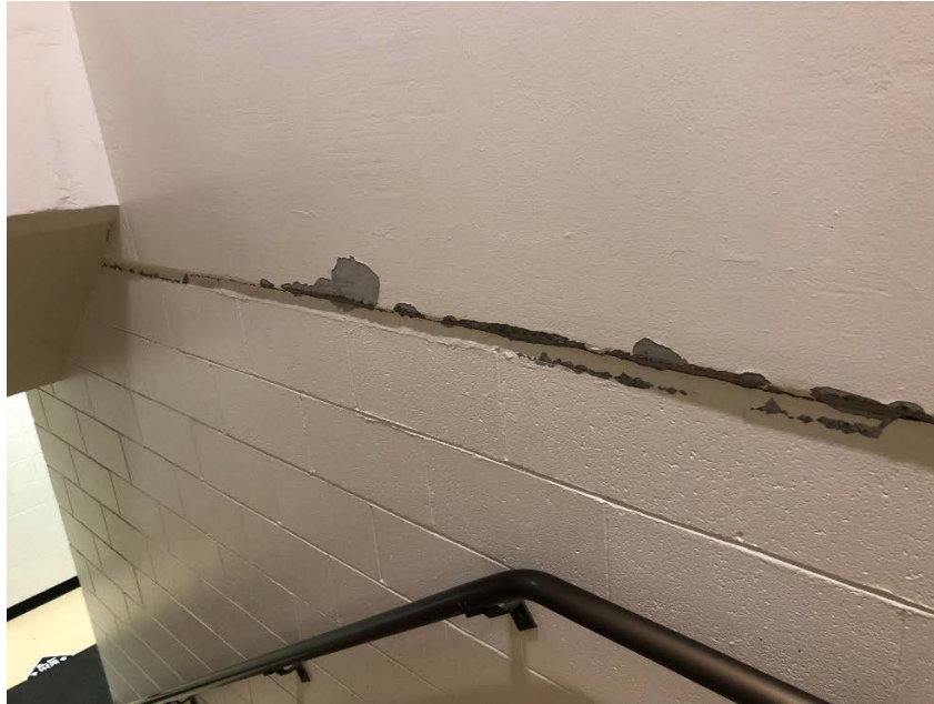
SW-3, CMU Cracking Figure B- 69
