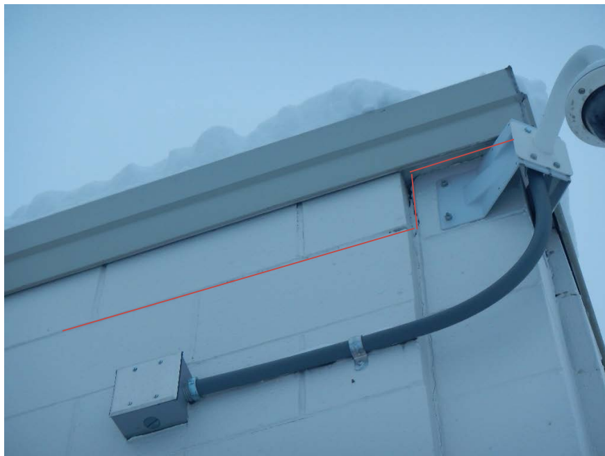
CMU Cracking Figure B- 8
