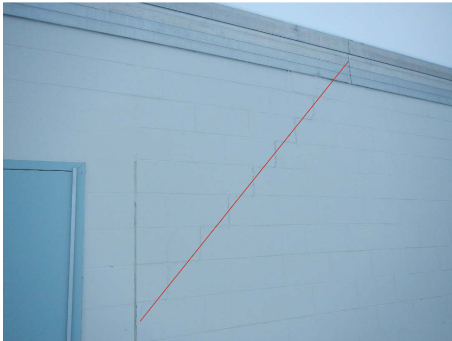
CMU Cracking Figure B- 10
