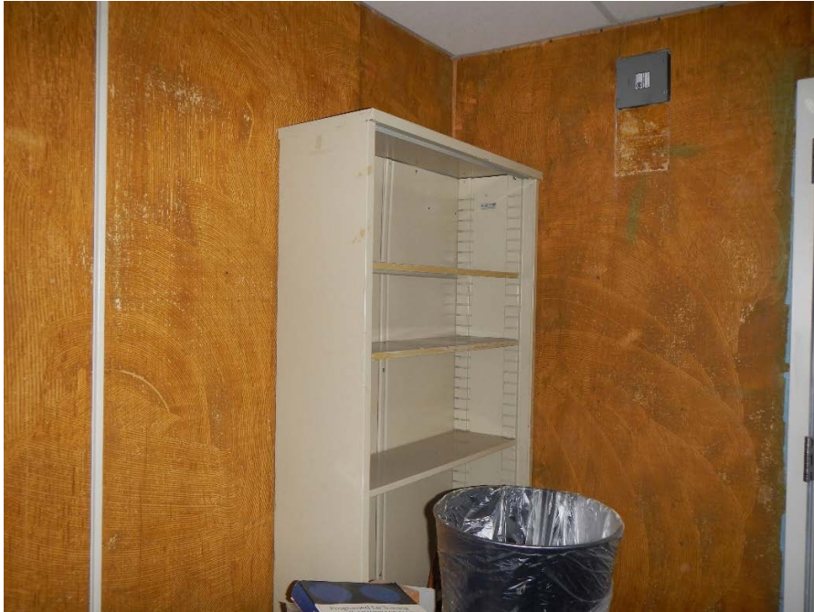
Room MO2C, Unrestrained Shelving Figure B- 17
