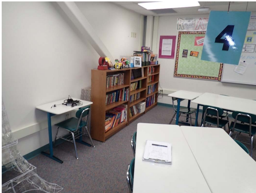
Room 145, Unrestrained Shelving Figure B- 20
