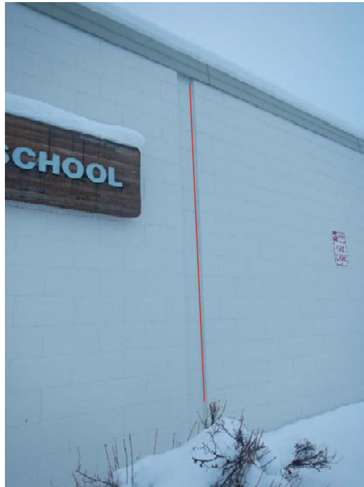
CMU Cracking Figure B- 7
