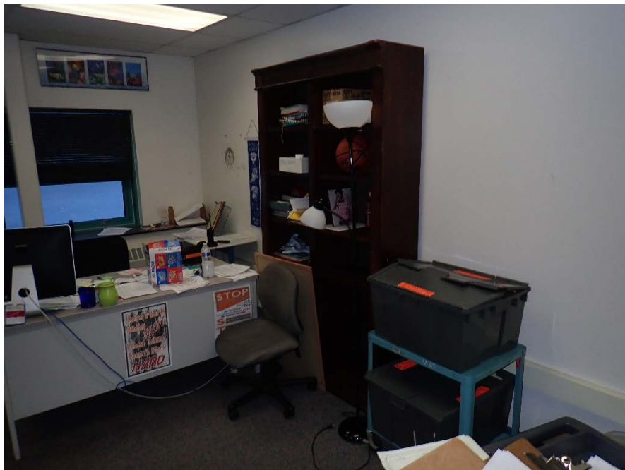
Room 143, Unrestrained Shelving Figure B- 21
