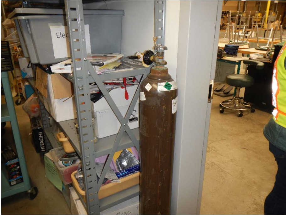
Room 105b, Unrestrained Hazardous Material Figure B- 34
