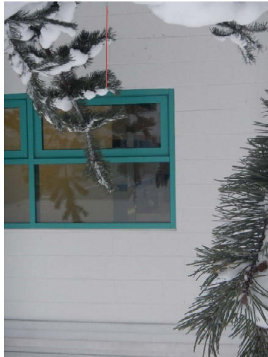
CMU Cracking Figure B- 12
