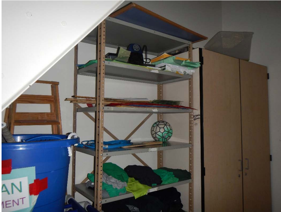
Room S07, Unrestrained Shelving Figure B- 15
