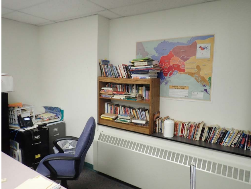
Room 138, Unrestrained Shelving Figure B- 25
