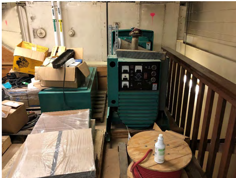
MCR Mezzanine 236, Fall Prone Contents Figure B- 58
