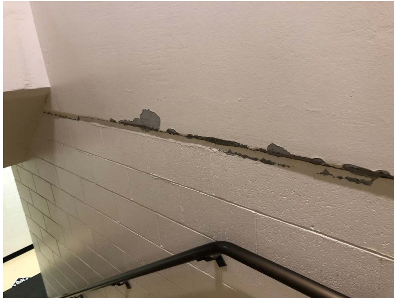
SW-3, CMU Cracking Figure B- 69
