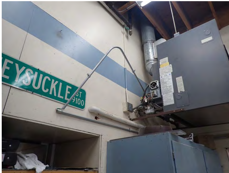
Glass Shop, Improperly Restrained Mechanical Unit
