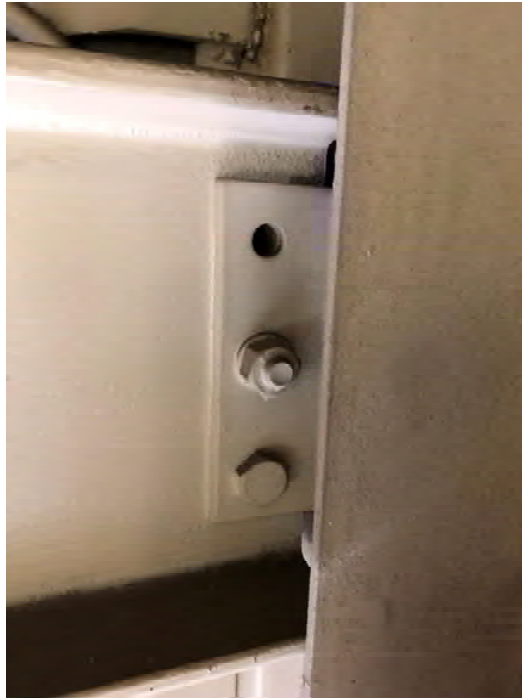
Vehicle Shop, South Bay Door, Header Missing Bolt Figure B- 47
