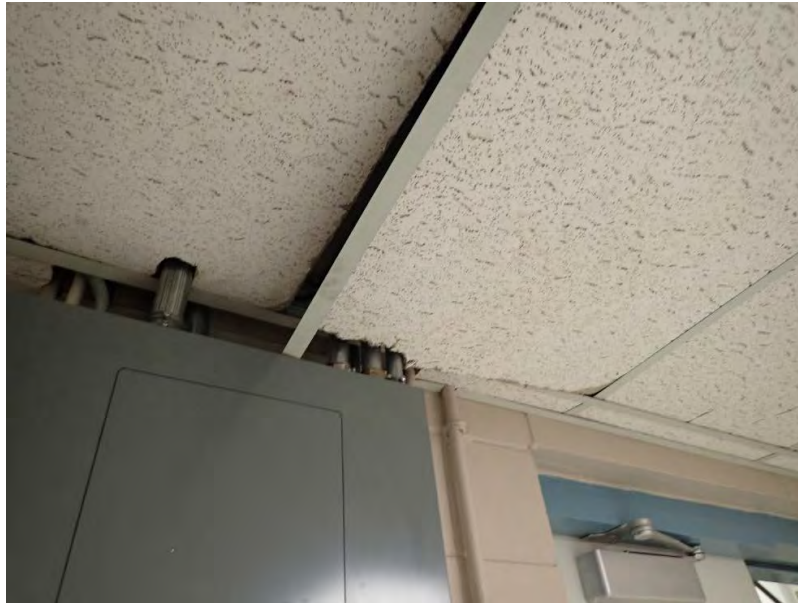
Corridor 150, Lack of Edge Clearance, Damage Figure B- 23
