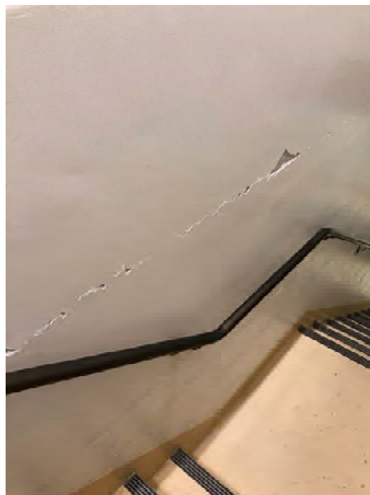
SW-3, CMU Cracking Figure B- 68
