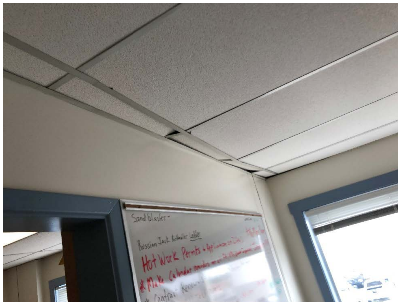
Regulation Room 242, Lack of Edge Clearance, Damage Figure B- 74
