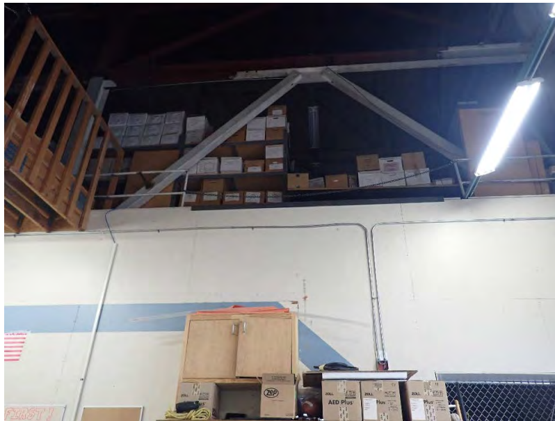
Glass Shop, Fall Prone Contents Figure B- 31
