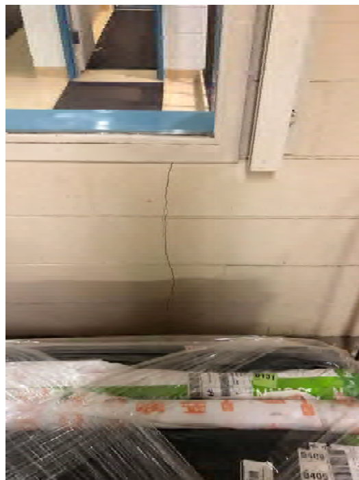
MCR Mezzanine 236, CMU Cracking Figure B- 62
