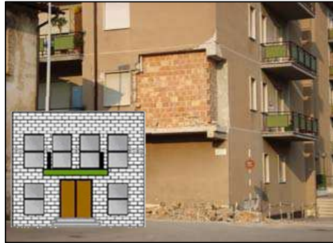
Figure 2: Immediate Occupancy (S-1) - Note damage to facade, but underlying structural brick in working condition.
