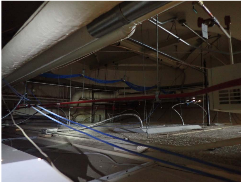
Corridor 150, Lack of Light Compression Strut Figure B- 25
