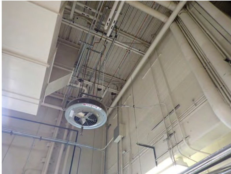
Room 105, Improperly Restrained Fan Figure B- 35
