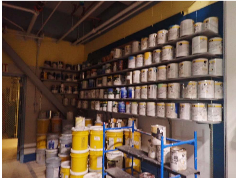
Paint Shop, Fall Prone Contents Figure B- 27
