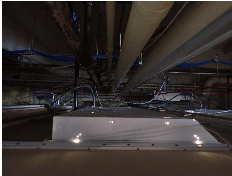
Corridor 150, Lack of Light Independent Support Figure B- 24
