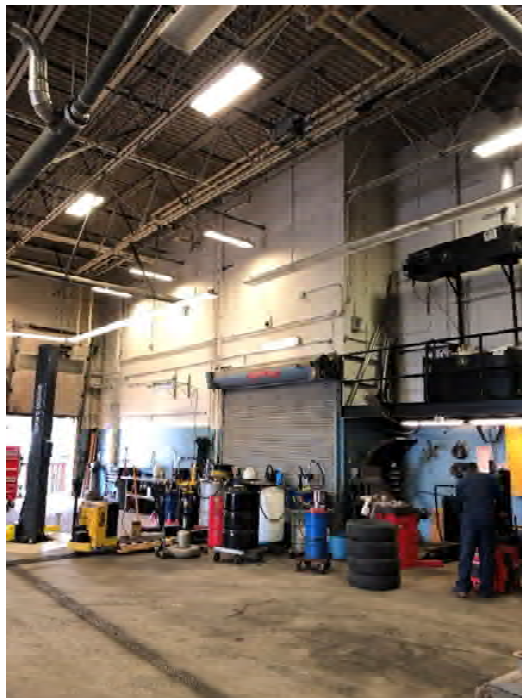
Vehicle Shop, Improperly Restrained Lighting Figure B- 48
