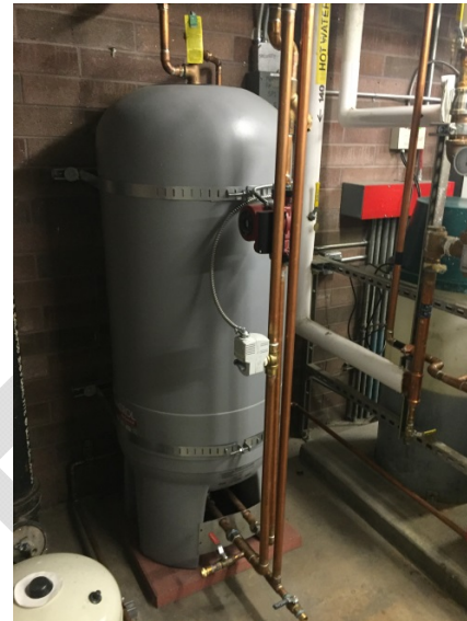
Original school area Hot water generator.
