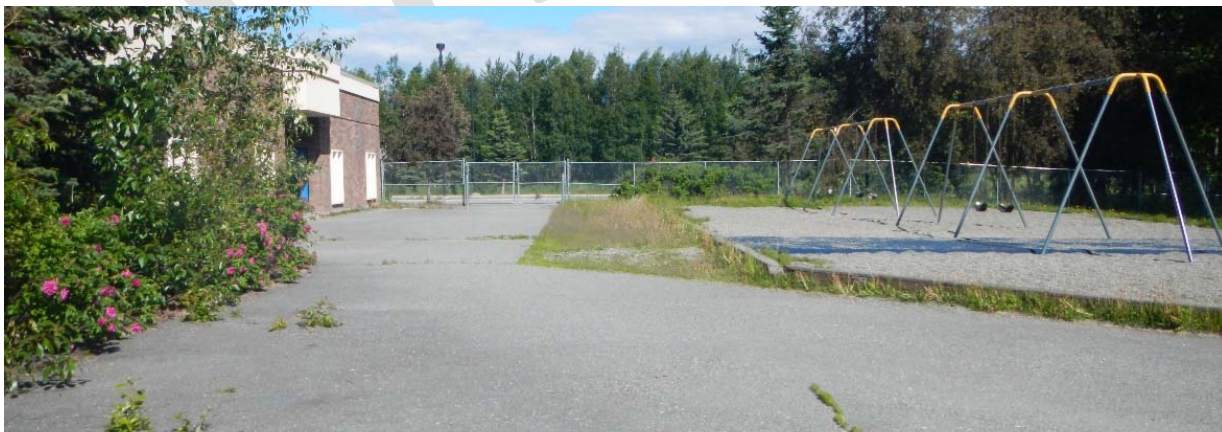
Hard Play Area Pavement Condition with Minor Cracking and Overgrown Vegetation
