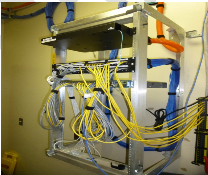
TR2 wall rack mounted in mechanical space
