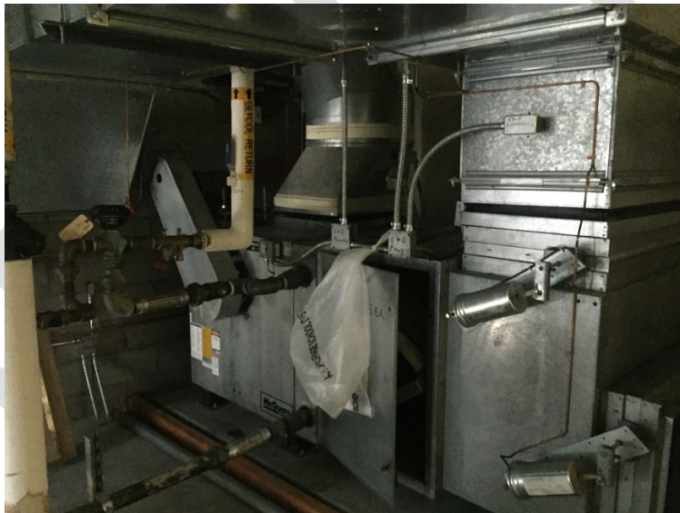
School addition AHU.
