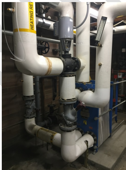
Glycol heat exchanger.
