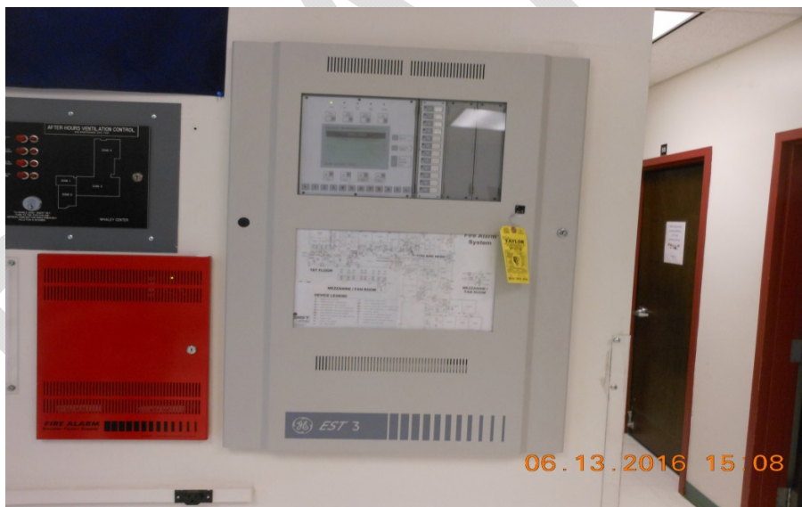
Fire Alarm Control Panel and NAC booster currently installed in the corridor. New system requires voice evacuation.
