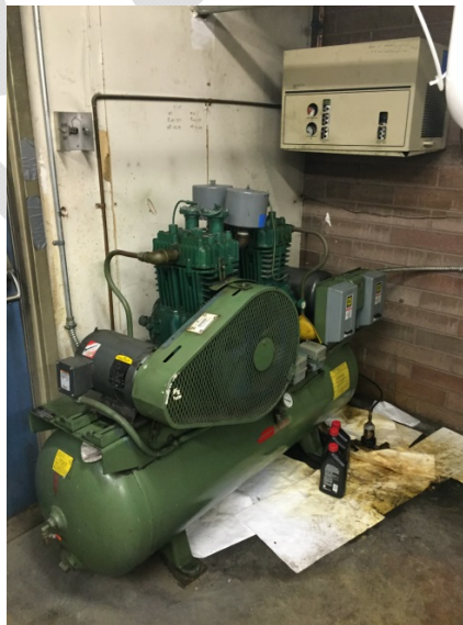
Control air compressor.
