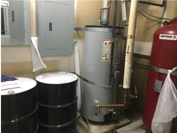
1991 addition Water heater.
