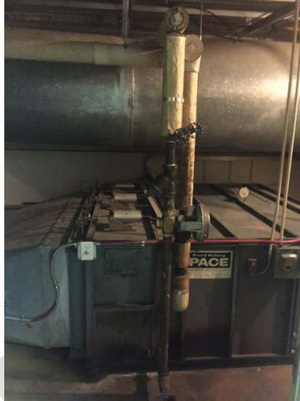
Multi-zone heating AHU.
