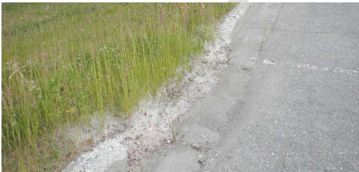
Existing Curb Cut in Pavement Area that has settled. Vegetation blocks drainage.
