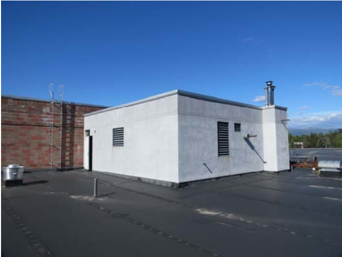
Existing Fan Room over the 1991 Addition.
