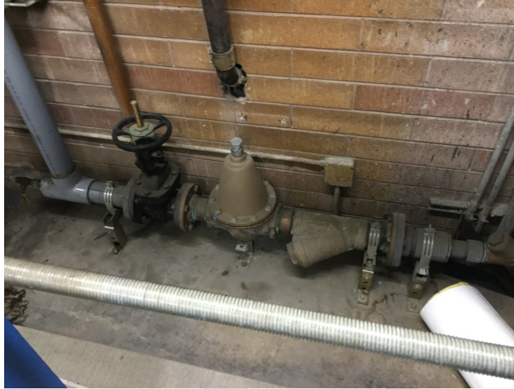
Water meter in the school addition mechanical room. Water meter for school addition is shown in school addition sprinkler riser photo.
