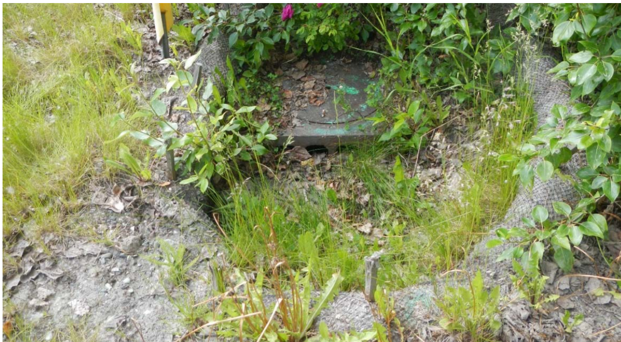
Existing Field Inlet on Northeast Corner of Site with Incorrect Casting and blocked by old erosion protection Measure
