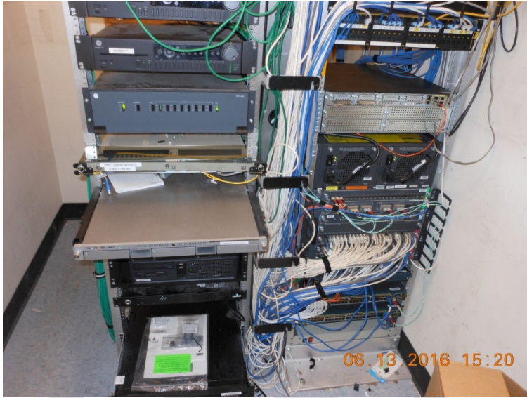
TR1 racks. Note width of room is inadequate to add any more equipment
