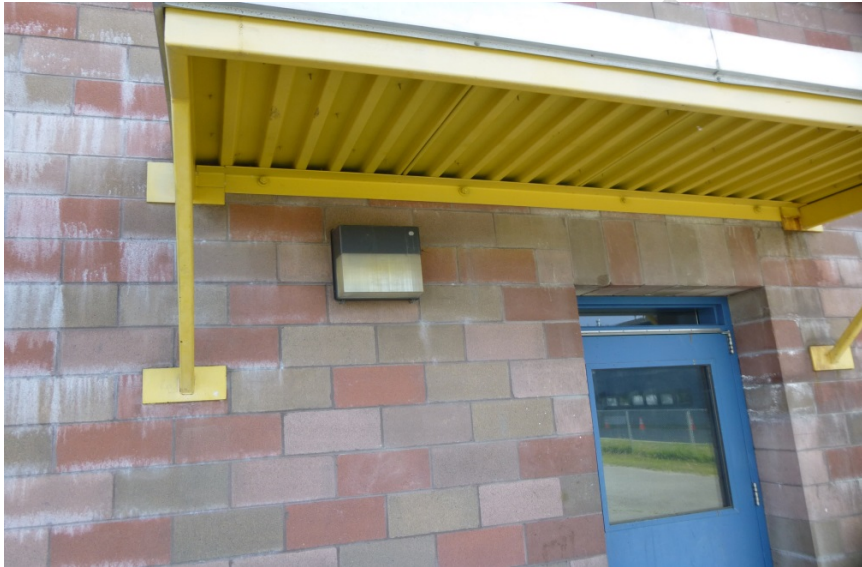
Example of aging exterior lighting
