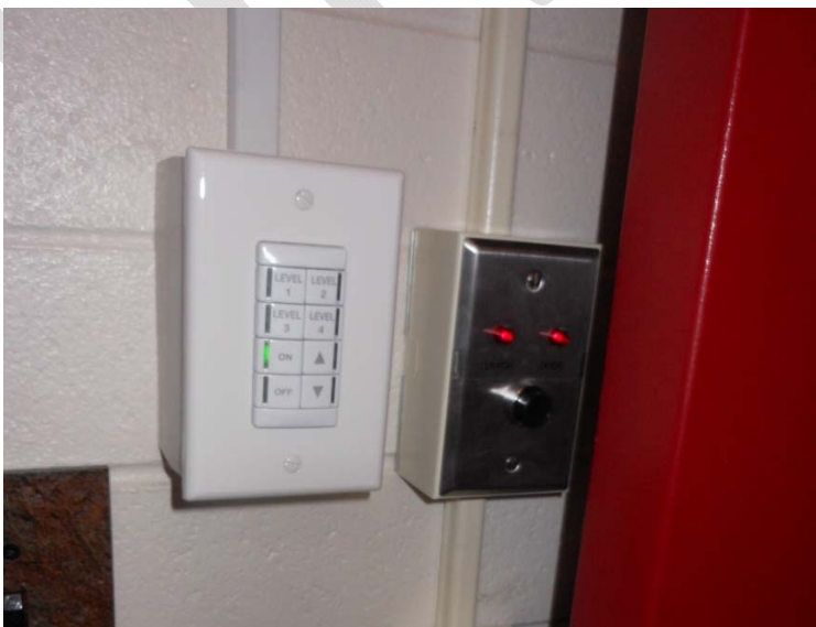
Lighting controls installed in office with the ability to program scenes for multiple zones of lighting
