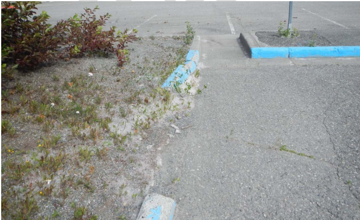
Severely Damaged Curb on North Parking Lot Island
