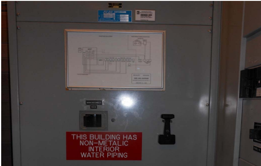
Existing service disconnect inside of the building is not compliant with current ML&P standards
