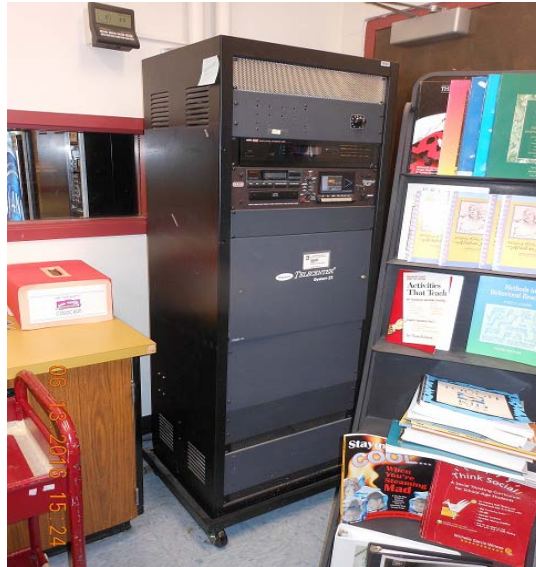
Intercom cabinet housing Telecenter 21 system, including cassette tape player
