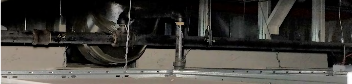
Figure 43 – Sprinkler heads without adequate clearance or flexible Line, typical of all locations.
