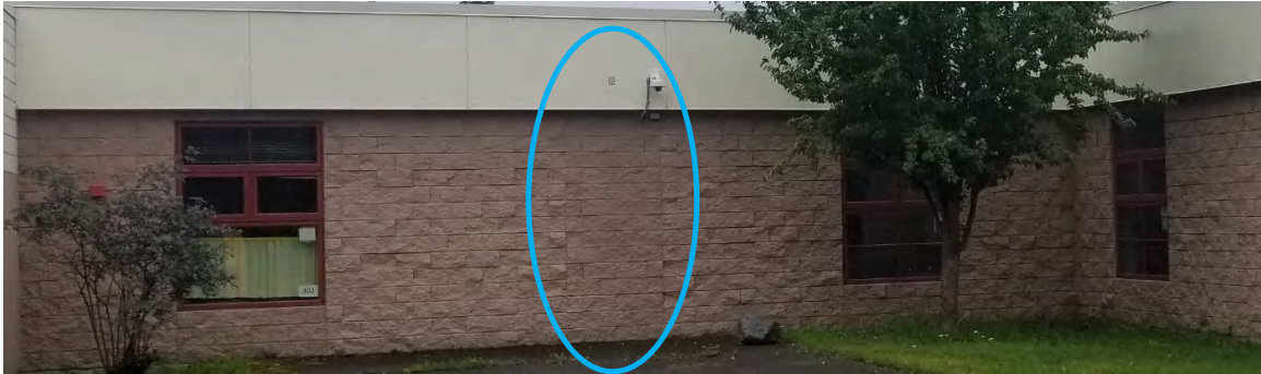
Figure 45 - Typical veneer attached to stud wall in previous opening without weep holes, occurring at various locations around the building. Photo location is at East side.
