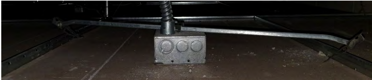
Figure 37 – Non-complaint bracing for emergency lighting above ceiling tile in corridor C-24.
