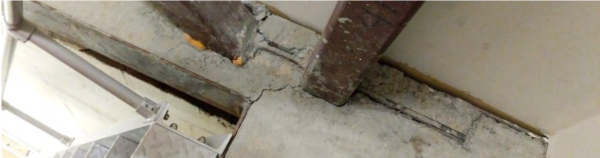
Figure 27 – Cracking in the slab on metal deck located near the stairway to the central mechanical penthouse.
