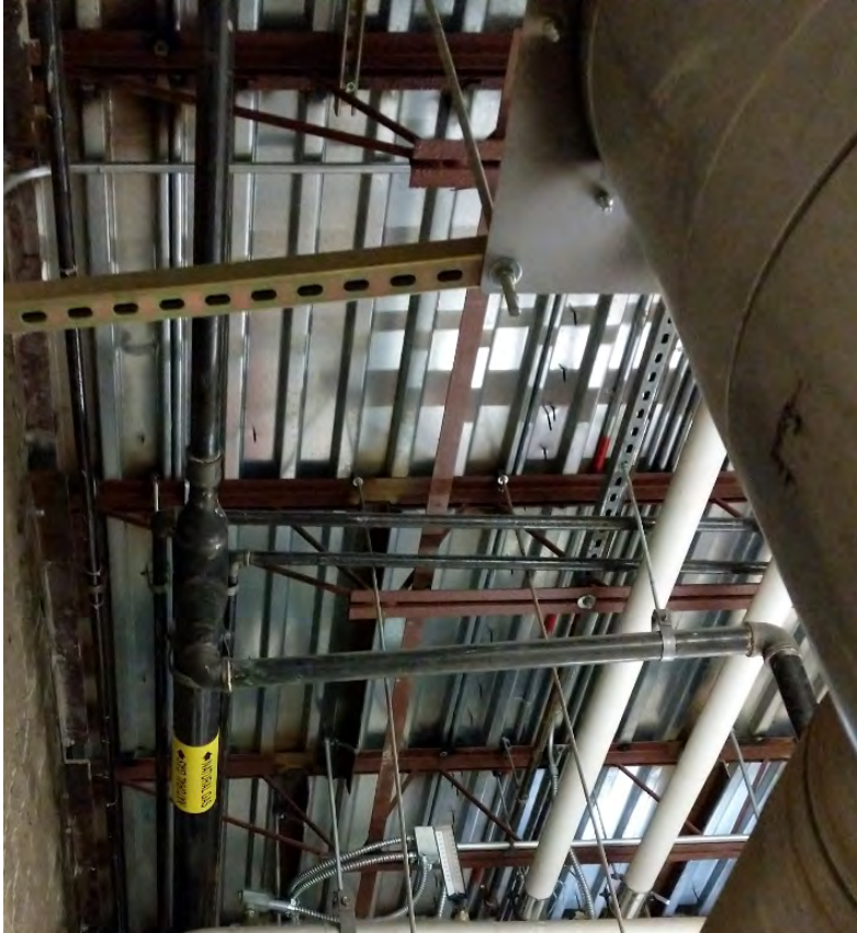
Figure 44 – Gas lines with no seismic bracing, located in the boiler room.
