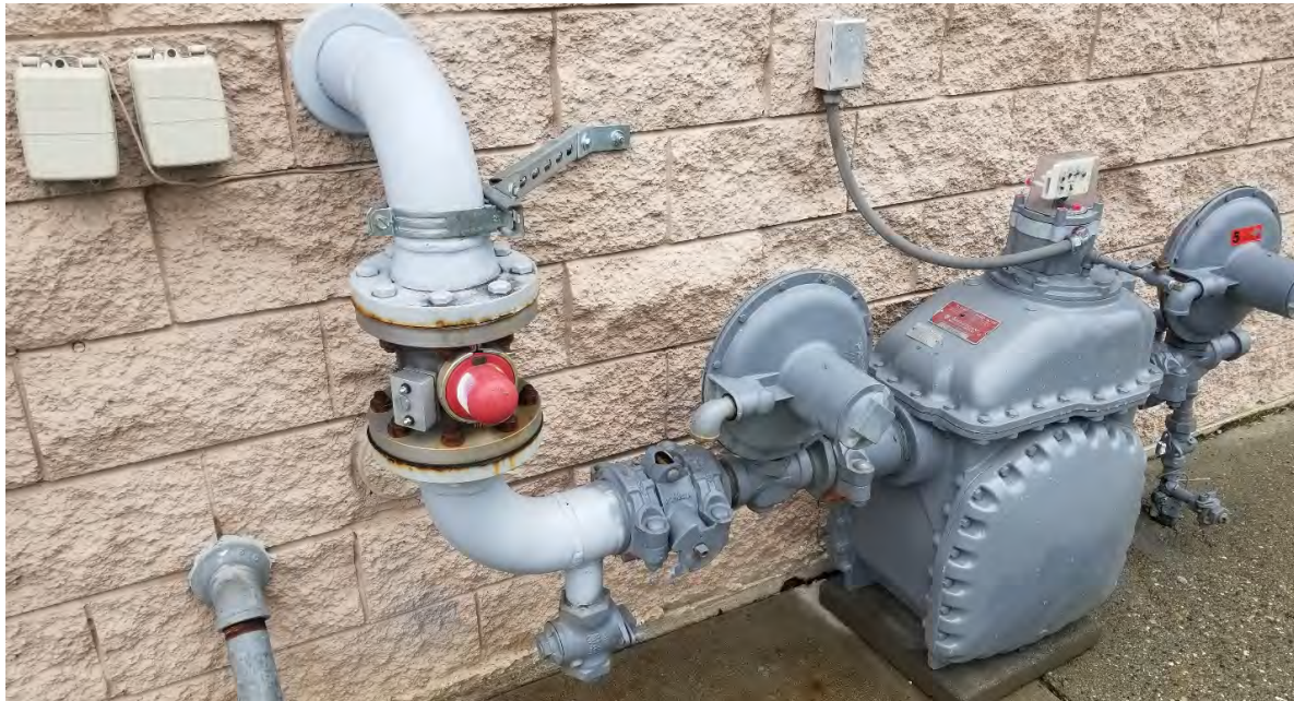
Figure 24 - Exterior natural gas connection to the building and seismic shut-off valve.
