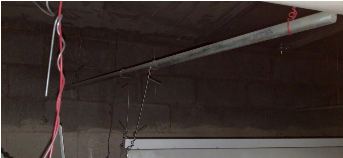
Figure 33 - Non-compliant light supports, above ceiling in corridor C-24.
