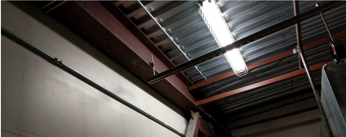
Figure 29 - C-clamps missing retaining straps at the new central mechanical penthouse.
