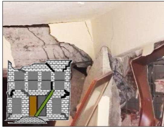
Figure 4: Collapse Prevention (S-5) - Severe buckling of members, near collapse.
