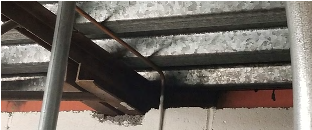
Figure 22 - Typical roof joist to CMU shear wall connection at the South mechanical penthouse.
