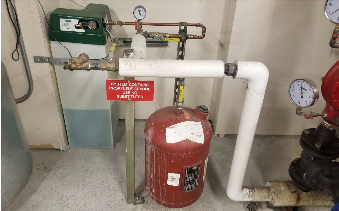
Figure 31 – Glycol expansion tank without adequate restraints, at the central mechanical penthouse.
