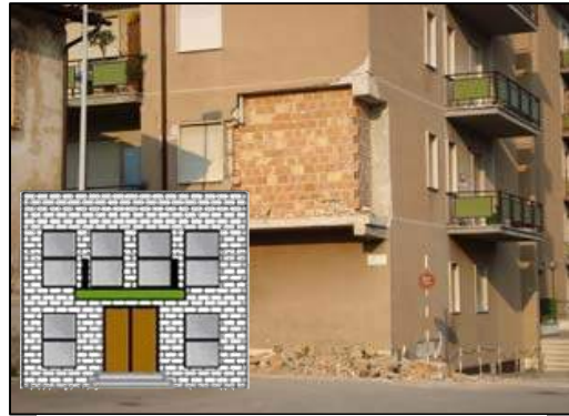
Figure 2: Immediate Occupancy (S-1) - Note damage to facade, but underlying structural brick in working condition.
