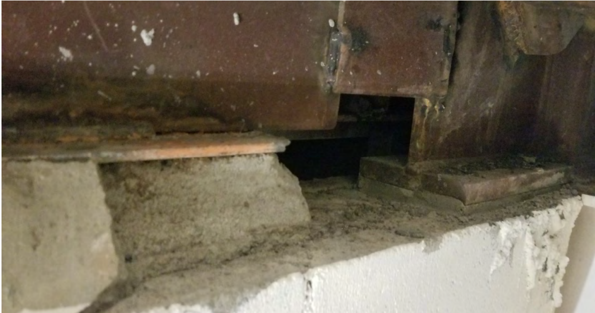
Figure 26 – Damage or incomplete grouting at the beam to CMU wall connection, located near the stairway in the central mechanical penthouse.
