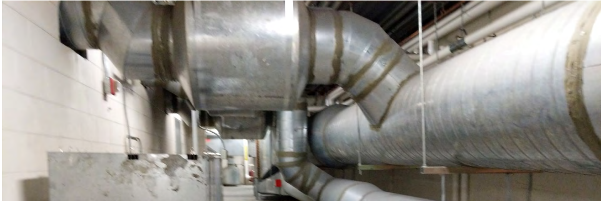
Figure 36 - Unbraced ducting, located in the South mechanical penthouse.
