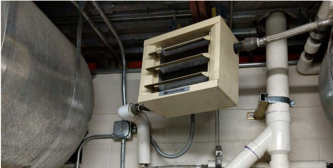
Figure 39 - Unbraced unit heater, located in the South mechanical penthouse.
