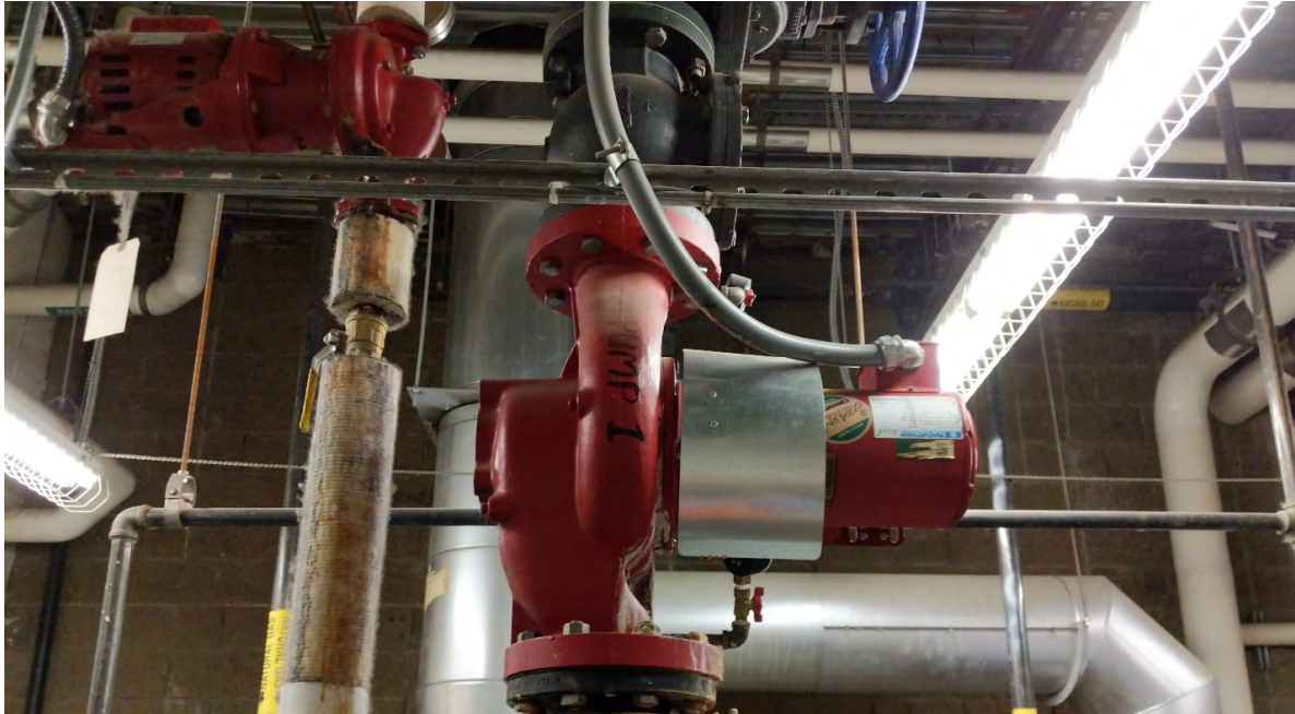
Figure 35 - Unbraced in-line pumps, located in the boiler room.
