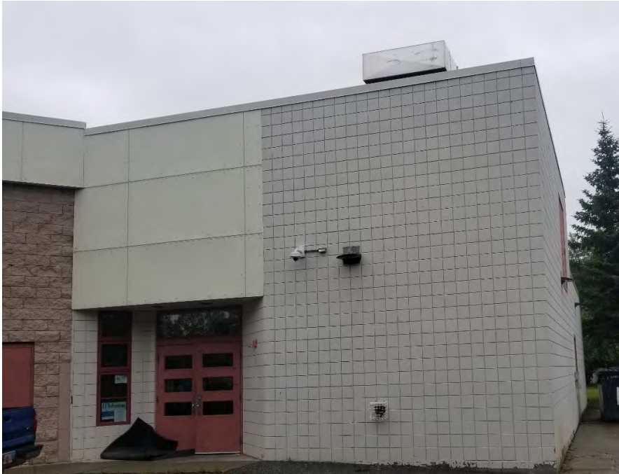
Figure 16 - South Mechanical penthouse and multi-purpose room.
