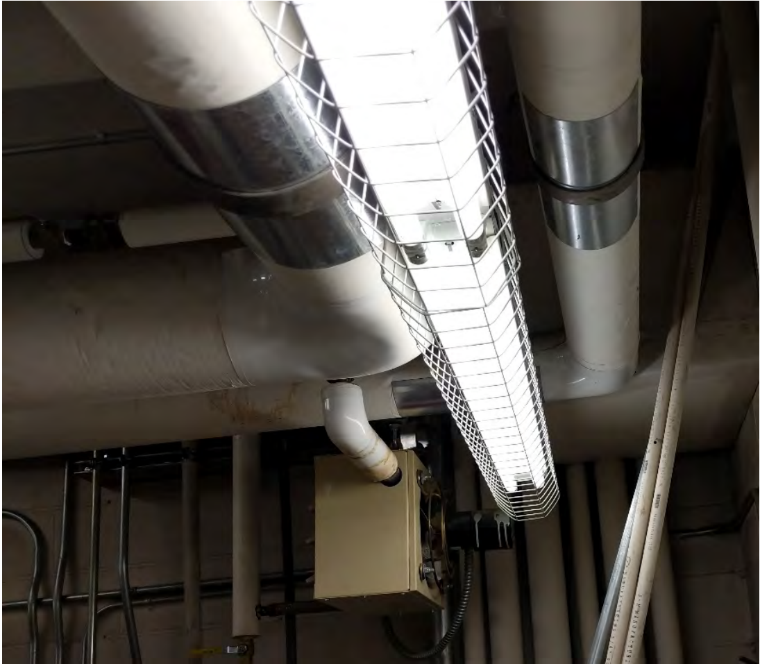
Figure 38 - Impact prone pendant lighting and unbraced unit heater, located in the sprinkler control valve room.
