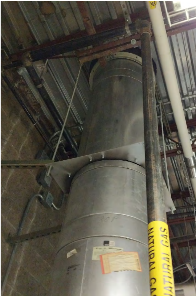
Figure 41 - Unbraced natural gas line, located in the boiler room.
