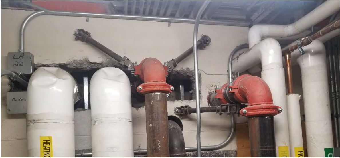
Figure 40 – Typical bracing at fire suppression piping mains.
