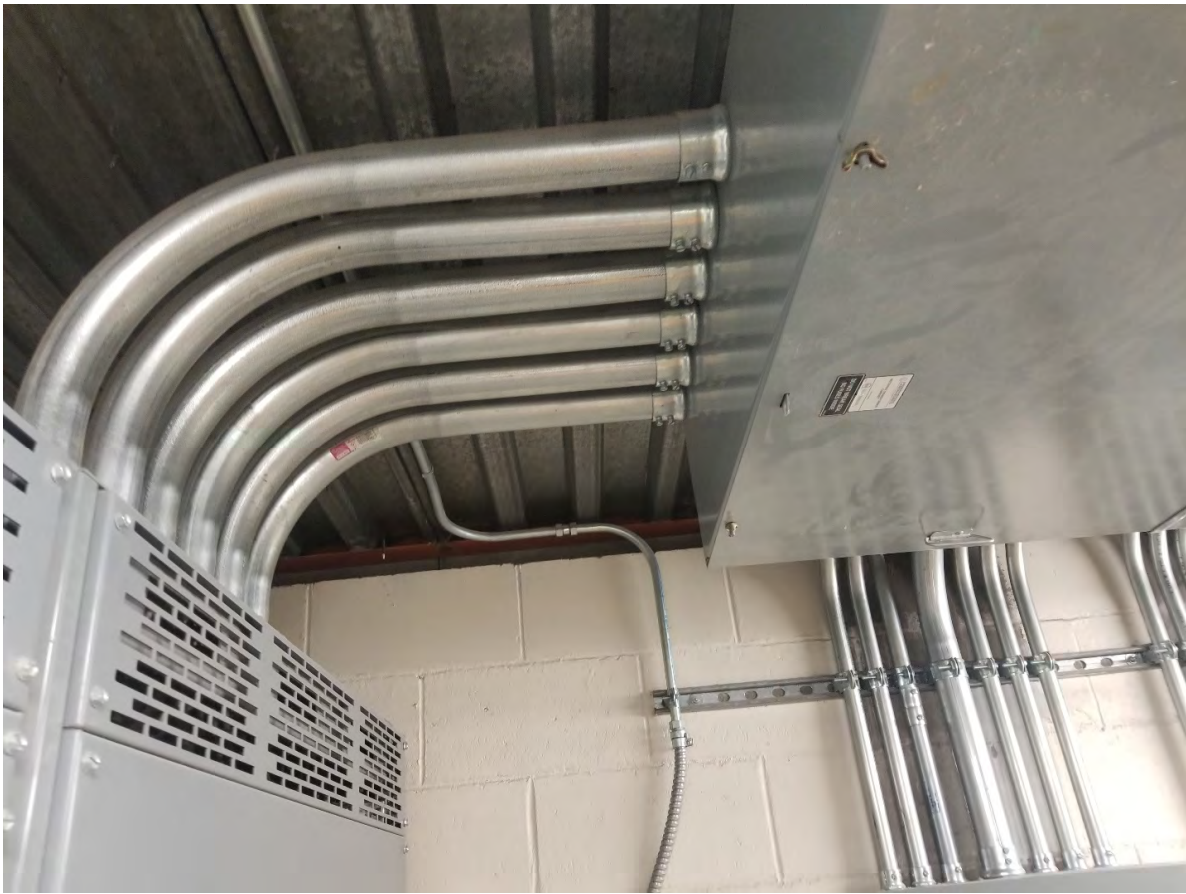
Figure 46 - Electrical conduit subject to relative displacements and lacking flex connections, located in the south mechanical room.
