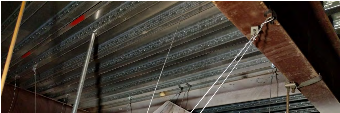
Figure 28 - Typical Ceiling Grid Bracing and typical C-Clamps with Retaining-Straps at wide flange beams.
