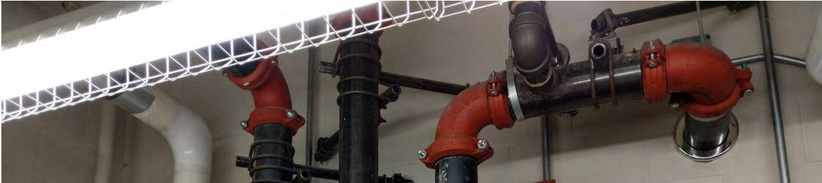
Figure 42 - Braced fire suppression mains, located in the sprinkler control valve room.
