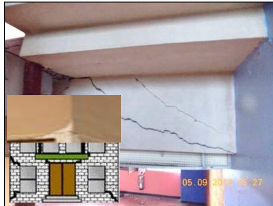
Figure 3: Life Safety (S-3) - Cracking/deflection in concrete beam, cannot be repaired.
