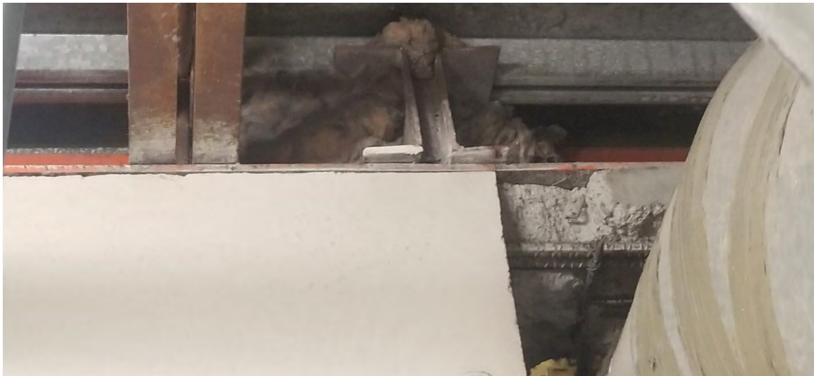
Figure 23 – Damage to the CMU shear wall in the South penthouse near grids H-7 of the 1999 Renovation and Addition drawings. Damage appears to be related to the installation of the mechanical duct shown in this figure.
