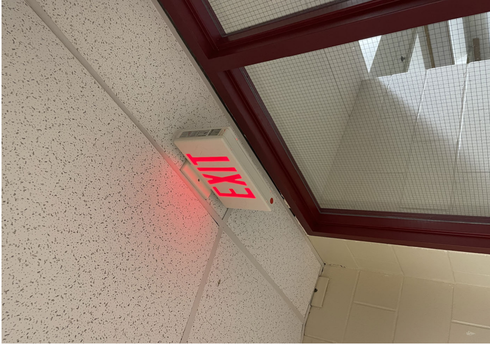
Exit Sign Self Test
