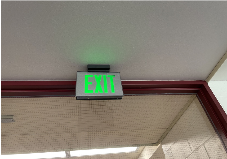
Exit Sign - Green
